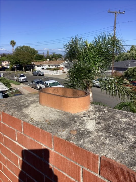
Missing Rain Cap
