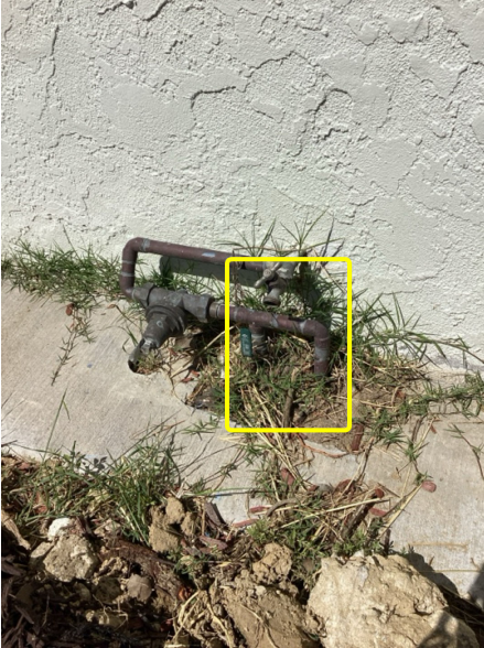
Main Water Shut Off: Left Side
