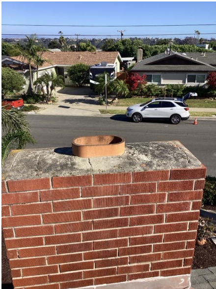
Missing Spark Arrestor
