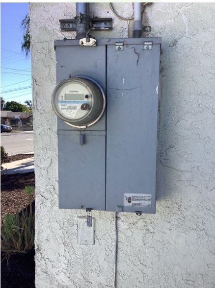
Main Breaker: Right Side
